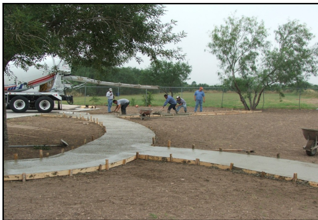
JIII Concrete lays the forms for the walkways which will connect the house with the Memorial Garden for family members and patients to enjoy.
